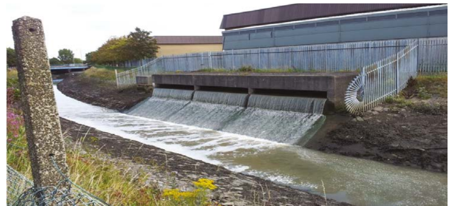
Figure 4.11 - Emergency Overflow at Sydenham WwPS
