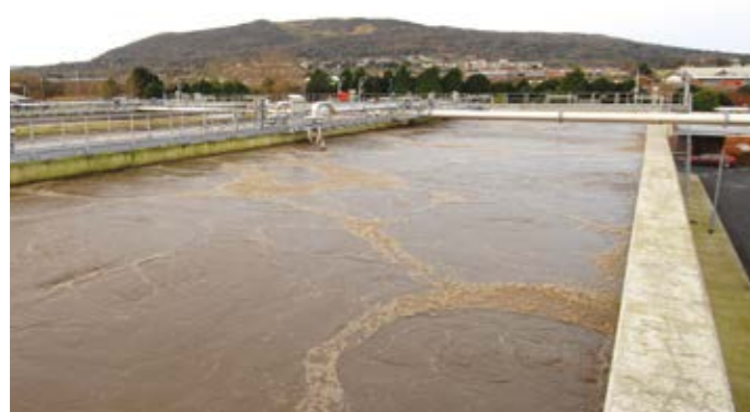
Figure 3.15 – Aeration Lanes at Whitehouse WwTW
