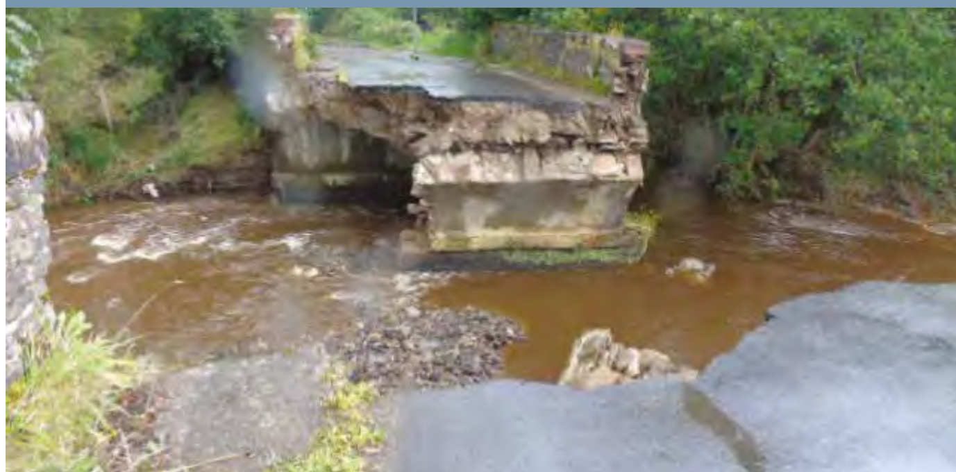
Figure 5.2-2: Collapse of the Glenrandal Bridge in Claudy (photo from NIFRA 2018) on the River Faughan, upstream of the Londonderry APSFR
