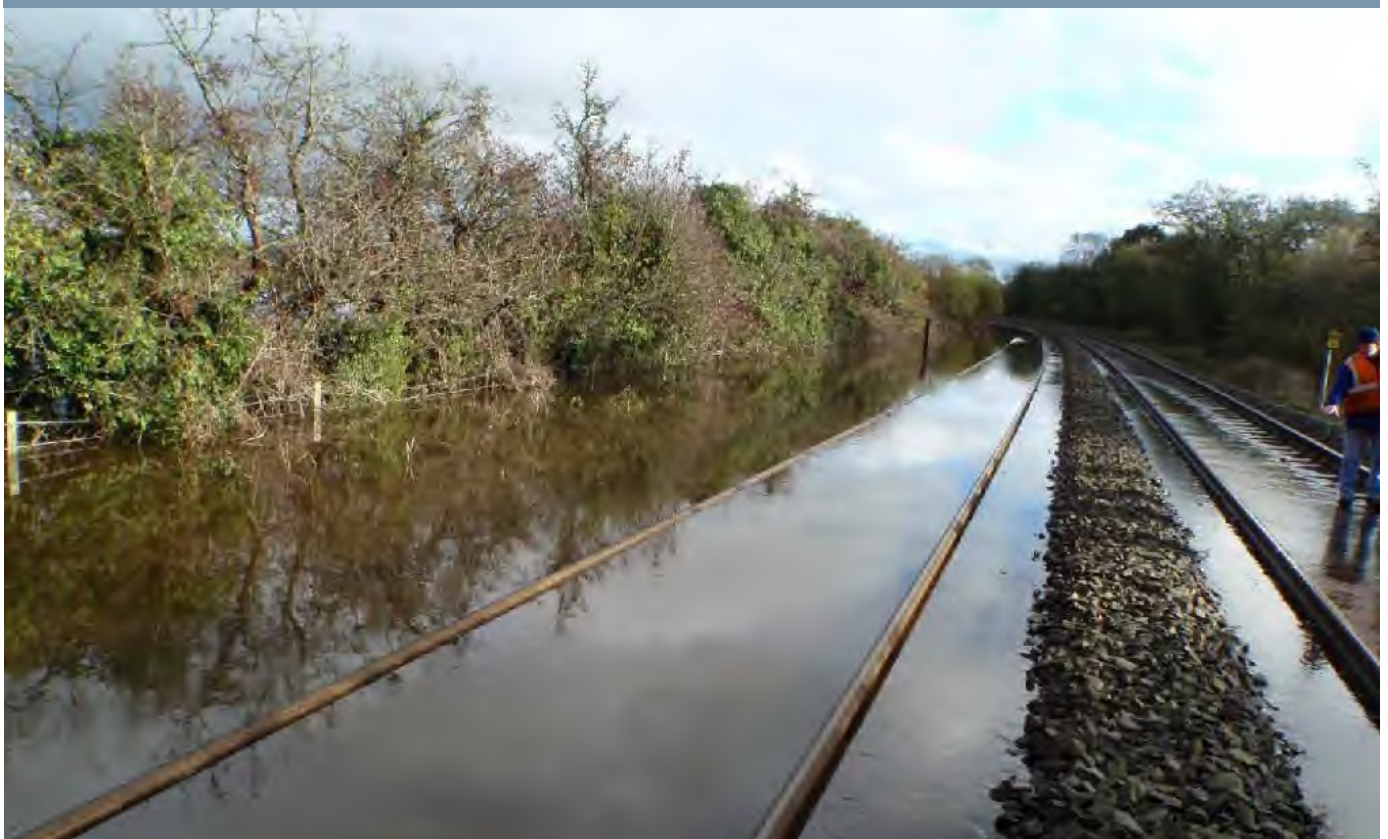
Figure 5.8-2: Flooding of the North/South railway line to the south of Portadown, October 2011
